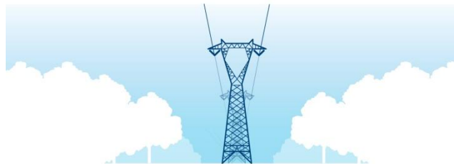
HVDC overhead line
