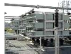
Series capacitor installation
