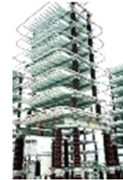
Capacitor installation for HVAV & HVDC
